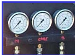
Pressure gauges. Park brake Accumulator Cable reel 3 x HYDEN264
